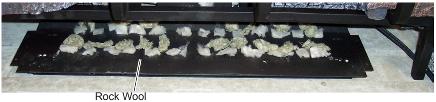
Figure 37 - Placement of Rock Wool (shown with Platinum Bright Embers)
